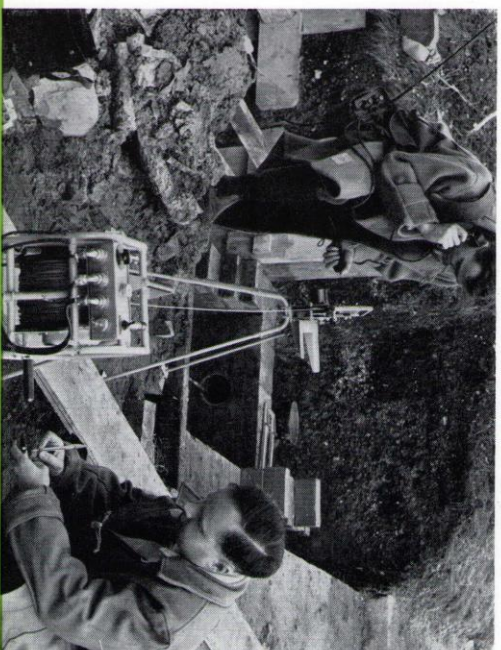
Using a radioactive technique to detect a leak in a water main.
